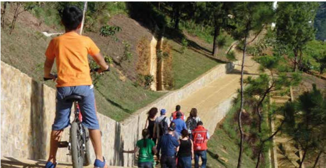
The beginnings of the Cinturon Verde (Green Belt) path. This 72 km project of pathways and landscaping trains employs local community members (mandated 30 per cent women) to build it. Its aim is to create a physical and psychological boundary to the city's sprawling growth and to connect and open remote communities. Offering magnificent views of the city, it should become a popular site for visitors. There are educational sites and eco-huertas (urban gardens) along the path. Image: Global Compact Cities Programme.
